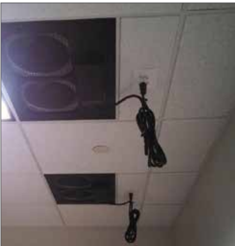
A ceiling-mounted air extraction fan.
