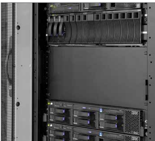
Use blanking panels to cover open u-spaces. This prevents hot air from recirculating back into the equipment inlets.
